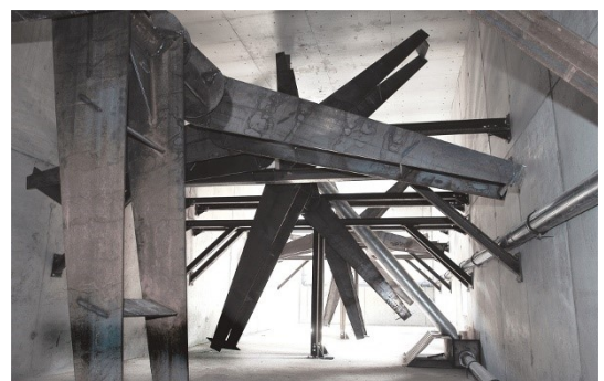
EUCO digester - Picture: Schmack Biogas GmbH
