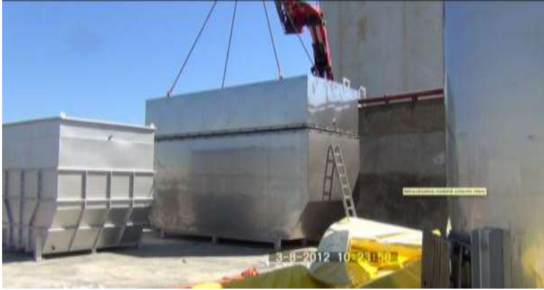
Anaerobic digester tank
