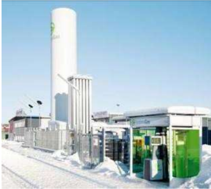
L-CNG filling station in Göteborg (Sweden)
